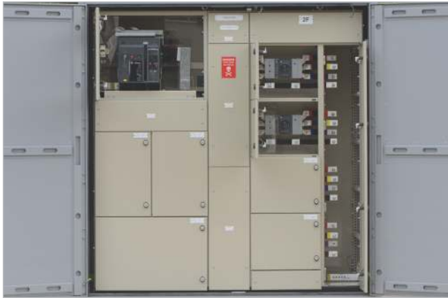
Figure 3.5: Low Voltage Compartment
