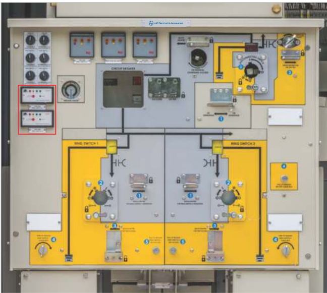
Figure 3.7.4: Fault Passage Indicators
