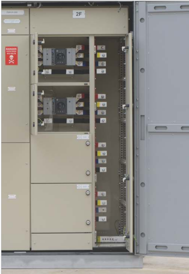
Figure 6.4.3 - LT Panel Cable Termination
